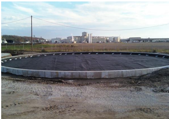
TANK RINGWALL – 60 MIL. HDPE LINER Provides leak detection underneath the floor of the tank as a secondary containment system.
